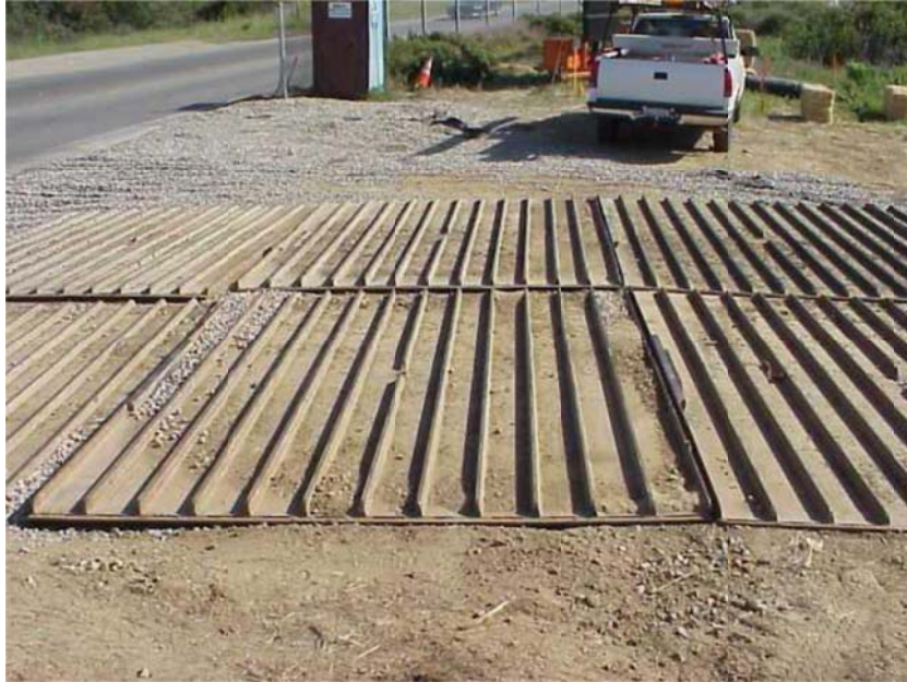
Manufactured metal plates knock dirt off vehicle tires before exiting a site.
